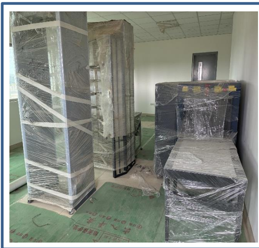
X-Ray Machine, Turnstile and Metal Detector Gate installed in Administration Building.
