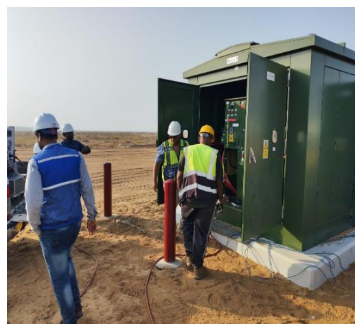
MV Package substation system testing
